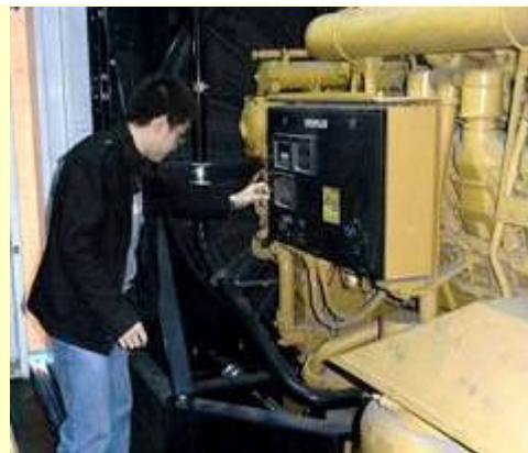
CEL staff ensuring rating meets load requirement
