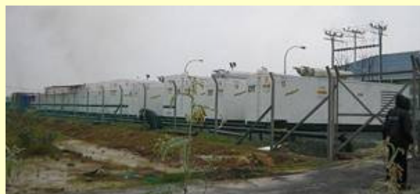
Close-up of SDI-supplied Cat power to SESB
