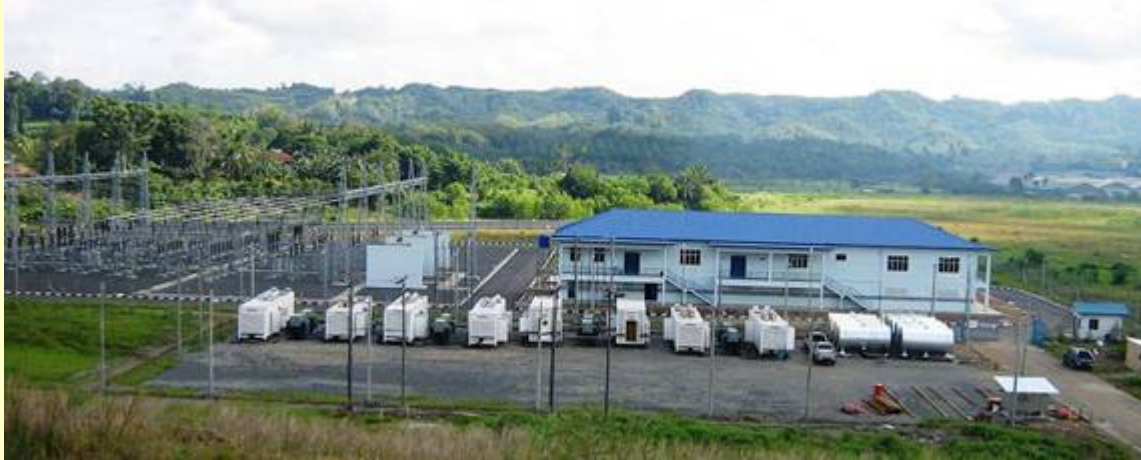
Reliable Cat gensets steadily providing power to the hinterlands of Sabah
