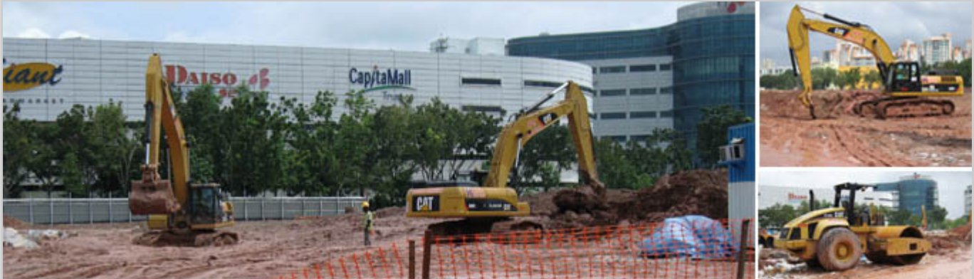
(Left photo) A pair of Cat hydraulic excavators working effortlessly in sodden conditions.
