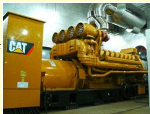
Cat C175, commissioned and ready to work at Hainan Telecom
