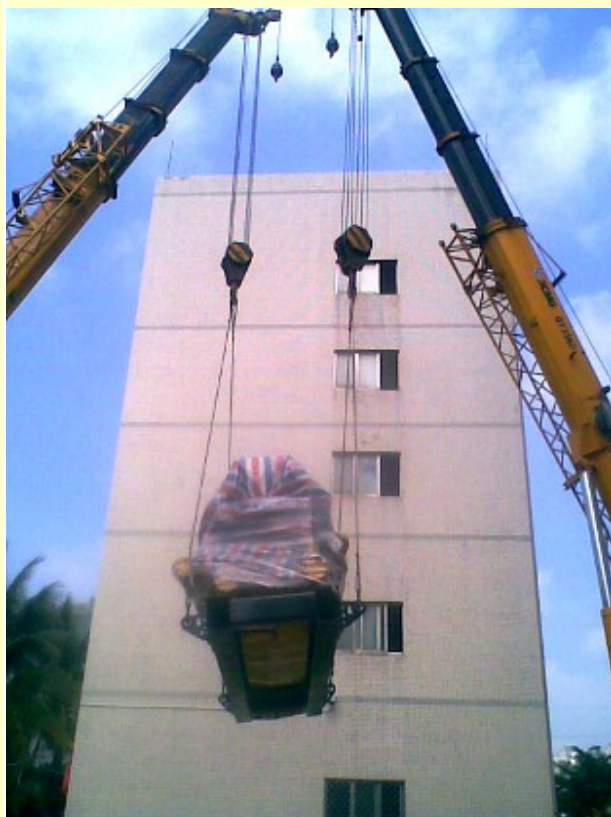
The Cat C175 on its way to its new home in Hainan Telecom's power room
