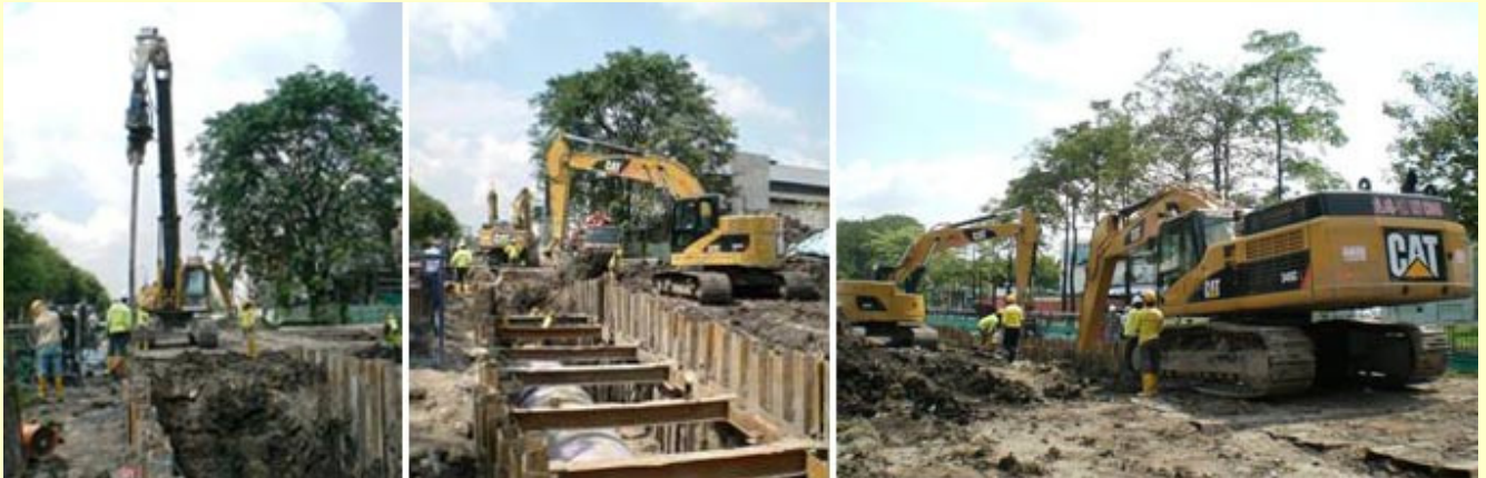
The Cat 345CL drives sheet piles into the ground. The Cat 321DL CR working in confined area.
